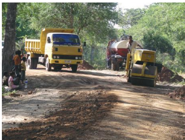
Figure 3. Road rehabilitation work in Timor Leste, using the equipment required for LBT.
