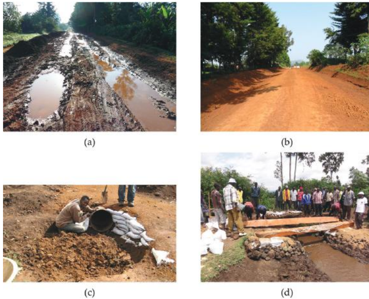
Figure 23. Applications of Do-nou technology during training/demonstrations with farmer groups: (a) Before construction; (b) after the construction; (c) retaining wall at inlet of culvert; (d) Do-nou abutment of wooden bridge.
