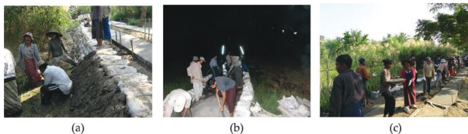
Figure 15. Construction at village K: (a) Covering Do-nou with clay; (b) working at night; (c) bucket brigade for casting concrete.
