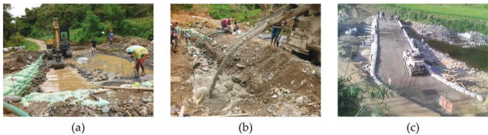
Figure 18. Work items managed using equipment provided by local government: (a) Excavation of the cut-off-wall and foundation; (b) transit mixers and water pump during casting concrete; (c) compaction of base course with roller.
