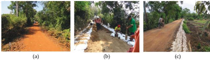
Figure 12. Construction of road embankment with Do-nou retaining wall: (a) Before construction; (b) construction of the embankment with Do-nou retaining wall; (c) after construction.
