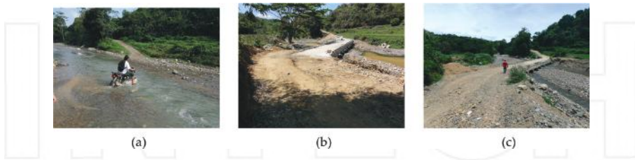
Figure 21. Conditions at the intersection with the river before and after construction: (a) Before the construction; (b) after the construction; (c) the conditions one year after the construction.
