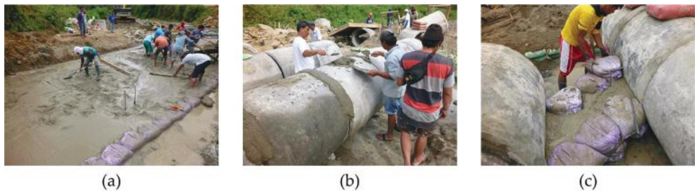
Figure 19. Work items managed by the community: (a) Leveling the concrete surface; (b) filling the gaps of RC pipes; (c) laying Do-nou.
