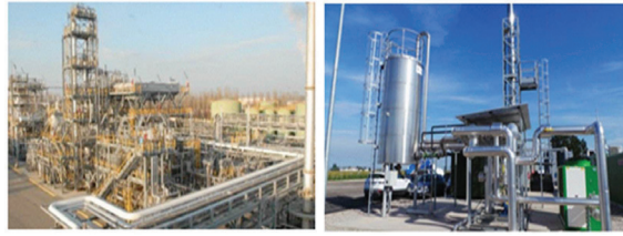
Figure 6. Chemical plant and hydrogen sulfide tank.
