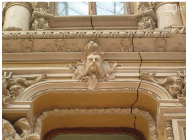
Pic. 4: Opened cracks on the facade of the "Passage"
