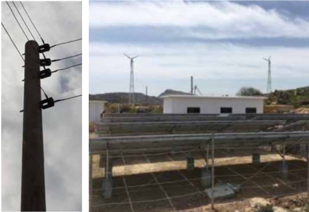
Concrete transmission pole at the Khushab site ( left ) and the solar PV-wind hybrid installation ( right ) at Khushab, Pakistan.
