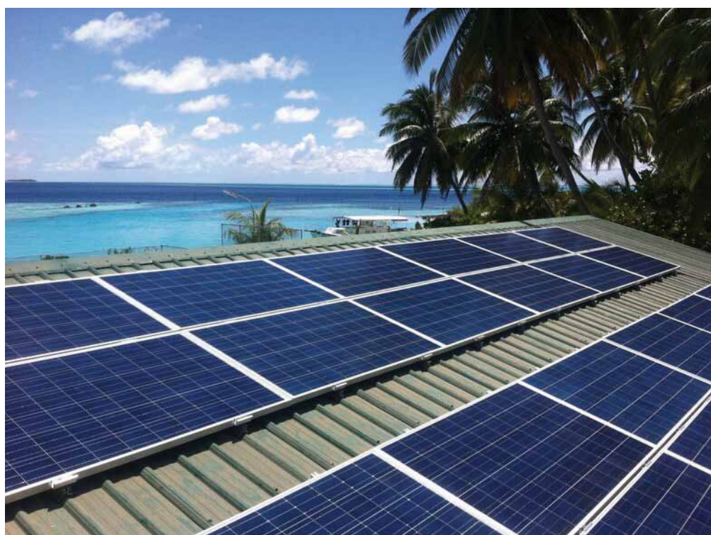
Photovoltaic Solar Power Plant on Rakeedhoo Island.
