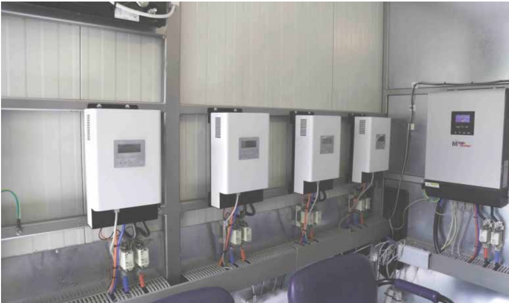
Compact Hybrid Power Plant at Power Development Board High School, Siddhirganj, Narayanganj, Electricity Company Bangladesh Limited.
