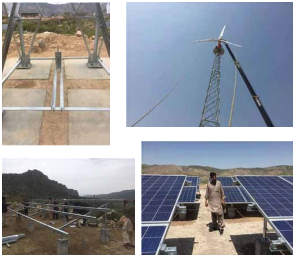
Clockwise from top left: Wind turbine tower foundation, installation of one of the small wind turbines, the fully built solar PV power plant at the Khushab pilot project site, and mounting structure for the solar PV array.
