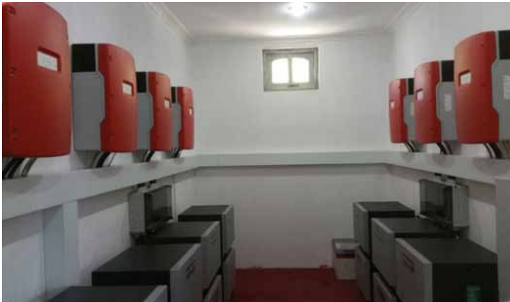
Solar photovoltaic array ( upper photo ), and battery bank and inverters ( lower photo ) in Dhihdhoo Island.
