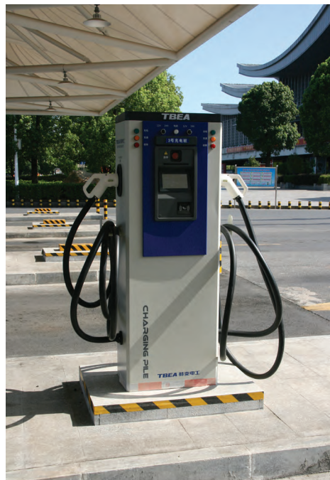
Charging station end-of-route for battery electric buses in the city of Hengyang, People's Republic of China.
