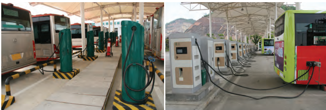
Chargers for battery electric buses in Tianjin (left) and Zhunyi (right), People's Republic of China. Source: Asian Development Bank.
