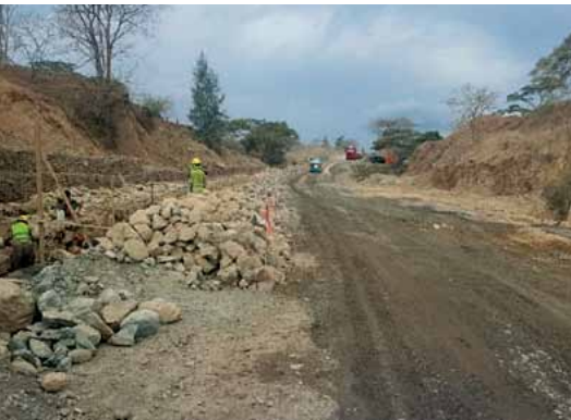
Top: Before construction, Station 45 + 794, Dili-Manatuto Road; Bottom: Same segment during construction, October 2017.
