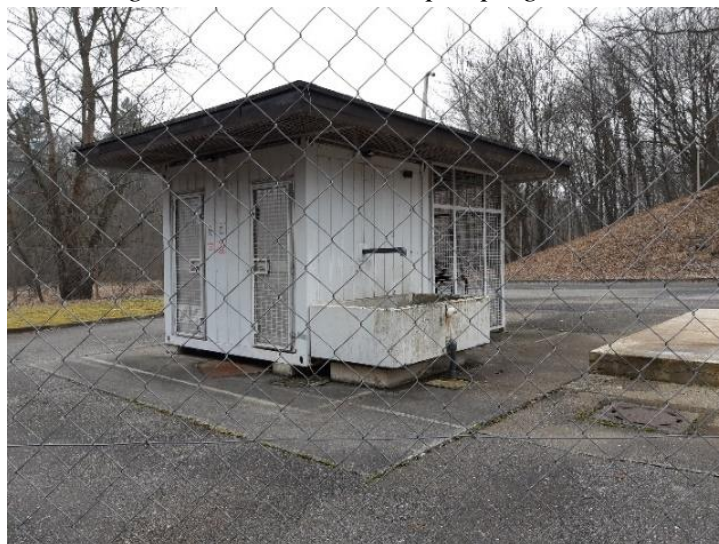
Figure 4: Thermal water pumping station
