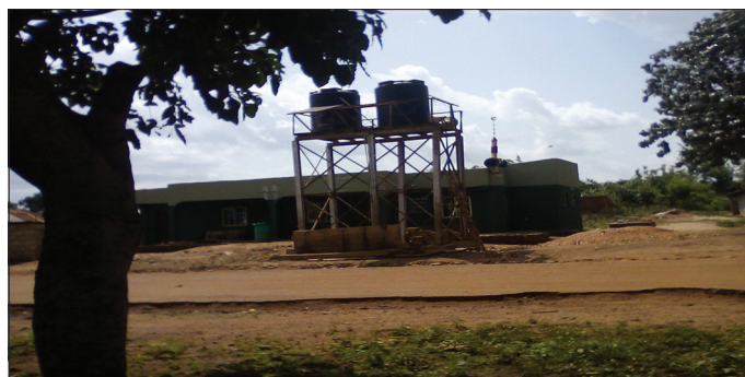
Plate 2: Solar-power water at Akodudu village (Atiba local government area)
