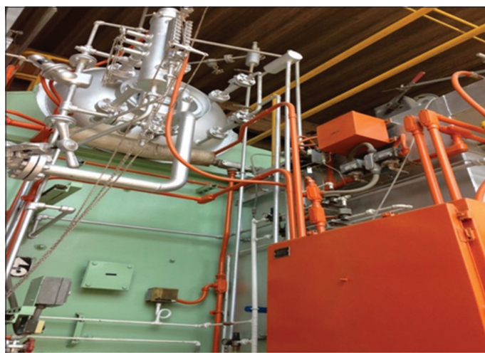
Figure 2: Boiler NEBRASKA BOLER COMPANY
