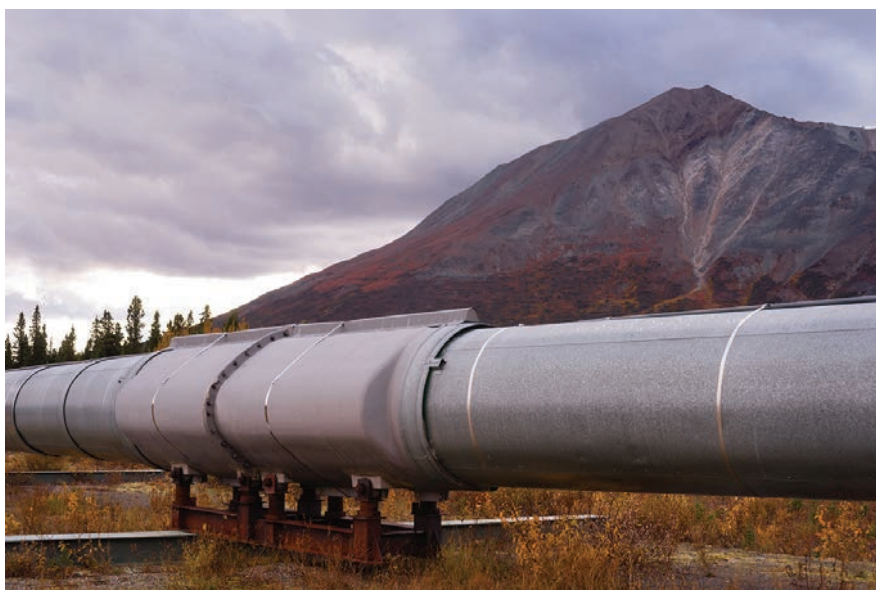
Pipelines in Alaska. Photo: Colorbox
