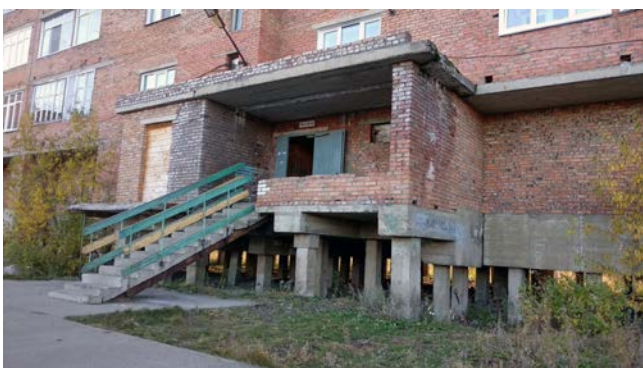
Figure 8.1a. The elevation of buildings (and other infrastructure) onto pillars allows for a ventilated layer between the structure and the ground, which helps protect against permafrost degradation: Igarka, Russia. Photo: Nadezhda Zamyatina
