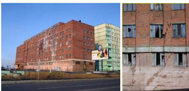
Figure 8.4. Building damaged by permafrost degradation, Norilsk, Russia. (Photo from 2013, now the building is dismantled). Photo: Nadezhda Zamyatina
