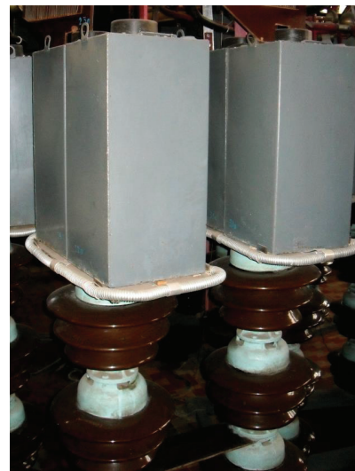
Fig. 4. Installation of IC-50-3 capacitors on support insulators to provide the necessary insulation from the ground in the impulse voltage generator
