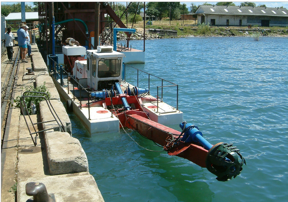
Figure 21: Small suction dredge and pilot wet mill behind for trial mining at Chipoka Bay in 2006.
