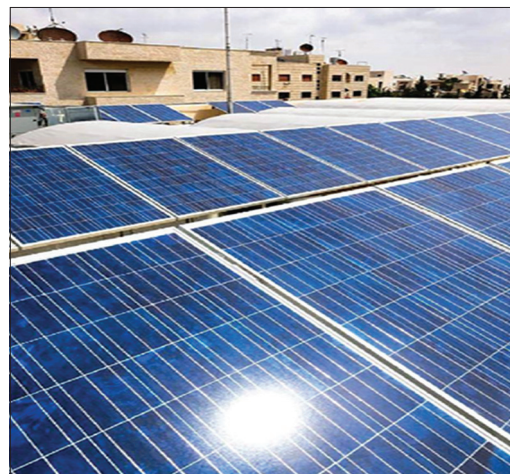
Figure 3: Solar panels implemented on the embassy's rooftop
