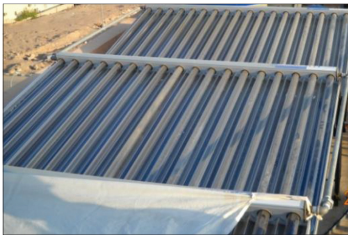
Figure 8: Solar water heaters installed at AR
