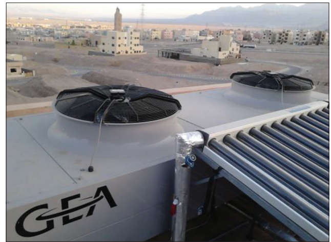
Figure 9: Dry Cooler installed at AR
