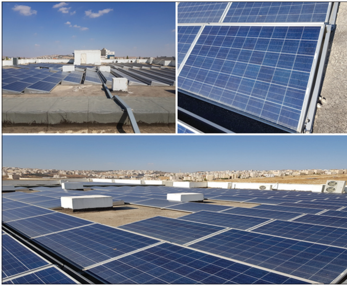
Figure 2: ASU PV panels
