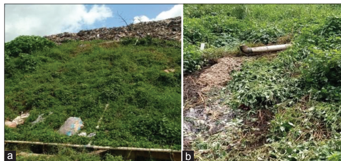
Figure 4: Capturing system of biogas (a) well gas (b) distribution pipe
