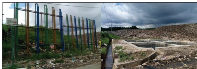
Figure 5: Flaring and leachate water treatment pool
