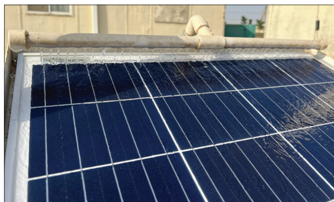
Figure 10: The water distribution manifold
