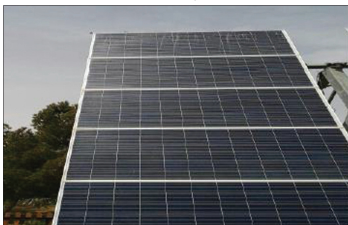
Figure 1: PV modules of nominal power of 285 Wp wired in series in one strings
